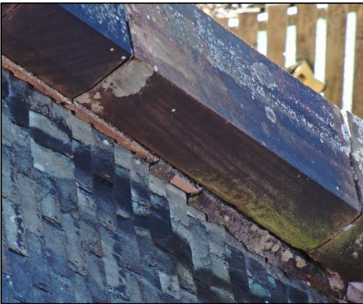
Missing/loose mortar skew and missing pointing between cope stones.
