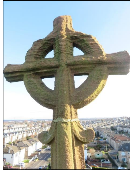
Our cross was inspected by one of the tenderers. Thankfully, while suffering bad erosion, it is stable and does not require major works.
